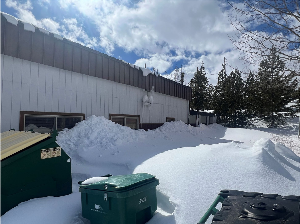
Image 4 Snow Pile Up on North Side of Site
