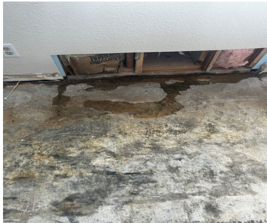
Image 3 Pooled Water on Inside of Site
