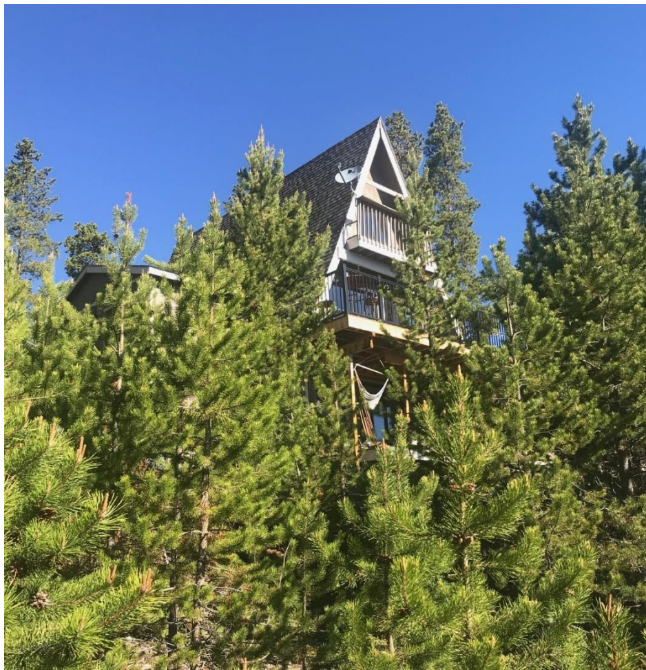
Rear of cabin showing slope issues
